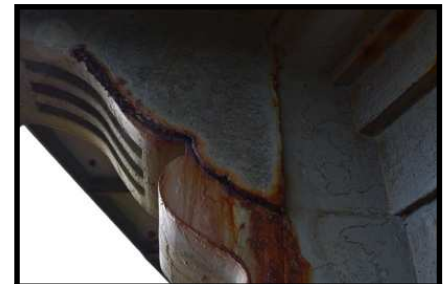
Rust damage on Bracket. Note crack, probably due to freeze jacking.
