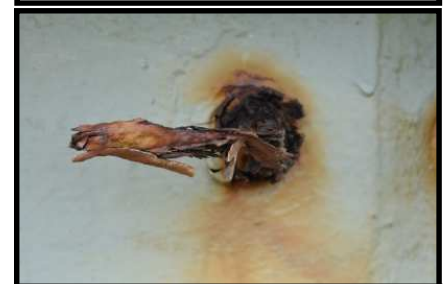
Remnants of a ladder rung above the lens room windows. These were used to support a portable ladder for window cleaning.
